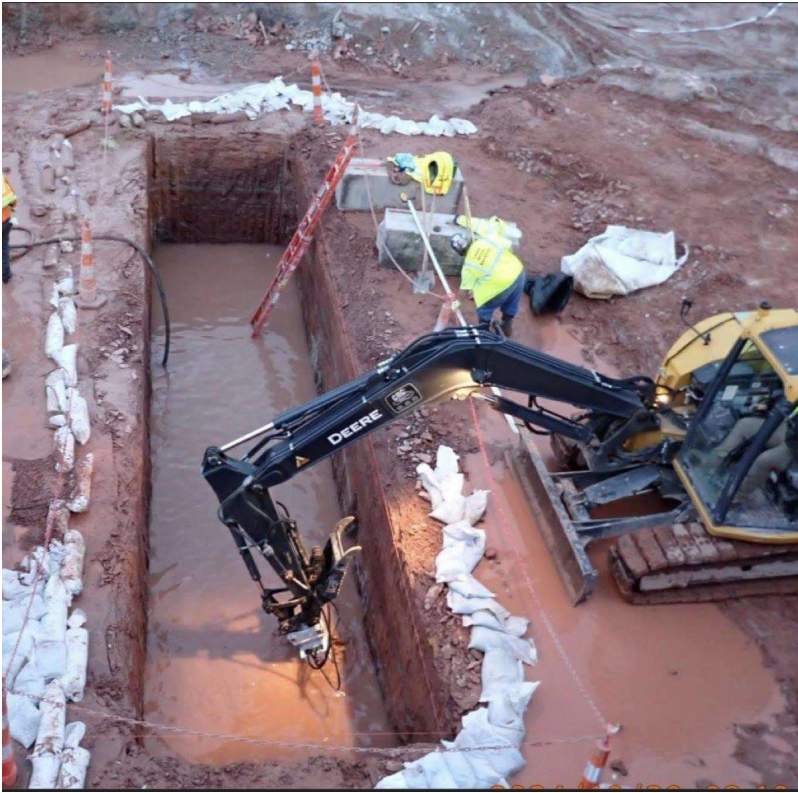
Excavation crews cutting into fill and bedrock (Jacobsville Sandstone) to create the foundation of the new and larger lock chamber. Credit: U.S. Army Corps of Engineers, Detroit District.
