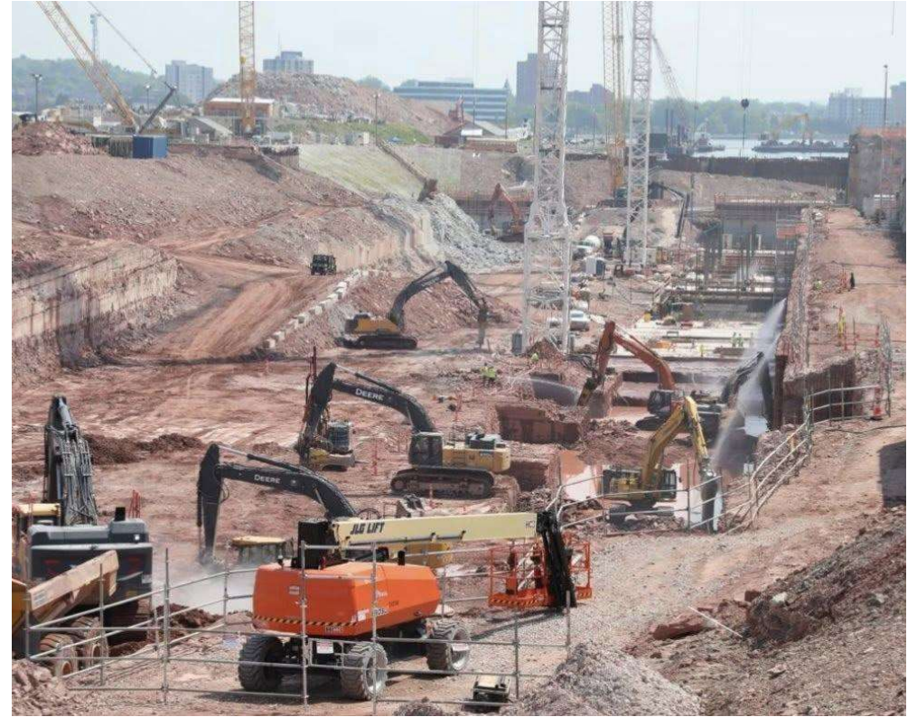
Heavy excavation exposes the underlying Jacobsville Sandstone as crews carve out the full length of the future 1,200-foot chamber. Credit: U.S. Army Corps of Engineers, Detroit District.
